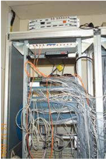
Rack A Switch
